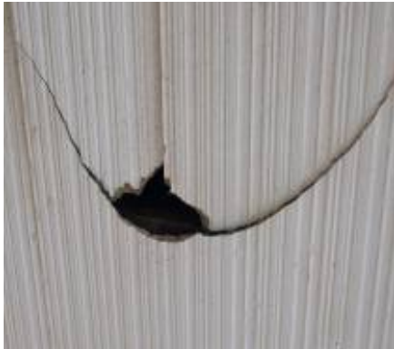
Photo 6: Examples of sharply broken edges on asbestos cement sheeting.
