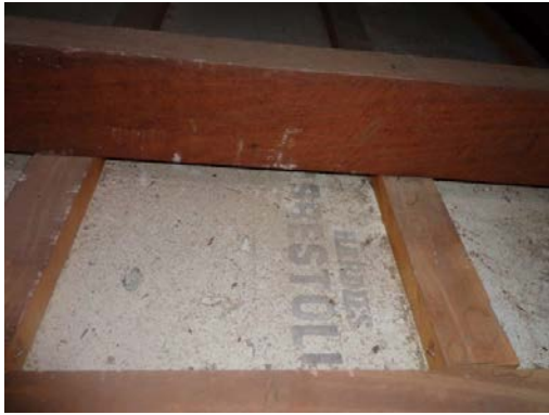
Photo 1: Rear side of LDB ceiling sheet showing trade name.
